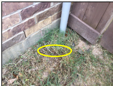
Ground rod does not appear to be fully installed into soil and/or improper ground clamp observed @ this time.
