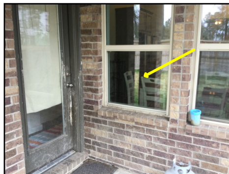
Window screen missing along breakfast room location
