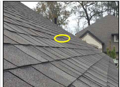
Debris/nails observed atop several exterior covering locations
