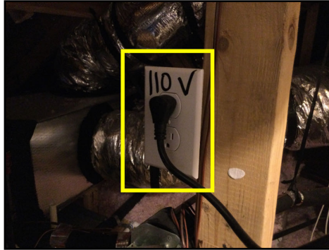
GFCI protection not established at attic support
