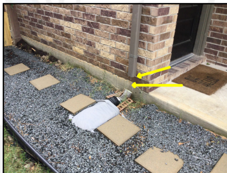
Gutter downspout elbow piping disconnected from vertical unit
