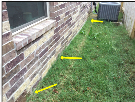
Soil to brick/siding contact observed along right exterior
