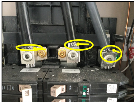
(Arrows) Anti-oxidant paste not present around service aluminum cables; (Oval) Cut/damaged wiring strands observed (Recommend an electrical contractor for further evaluation)
