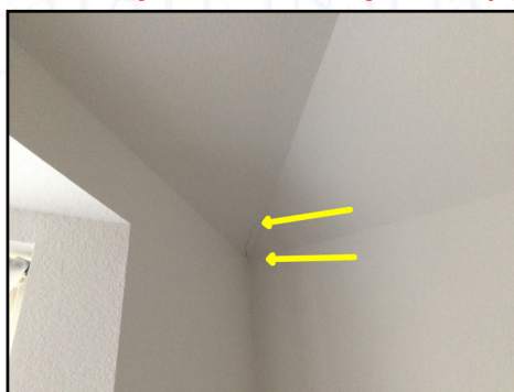
Drywall cracking observed along primary bedroom sloped scelling (There did not appear to be any signs of moisture intrusion or areas did not appear to be foundation related in my opinion)
