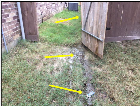
Water settling area(s) observed along one or more location(s) @ time of inspection (Recommend a landscape contractor for further evaluation across all areas to eliminate water settling)
