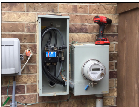
Right exterior disconnect panel inspected
