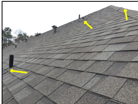
Lifted vent trim/shingles observed along right exterior
