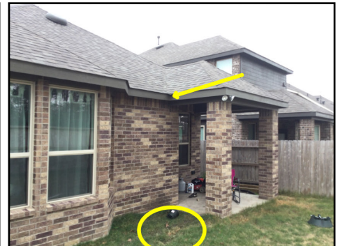
Water settling observed along back exterior soil under roofing valley
