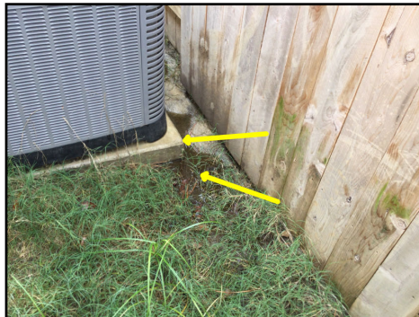
Water settling area(s) observed along right exterior swale.
