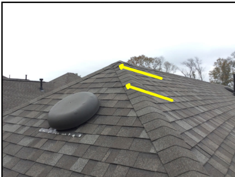
Lifted shingles observed along back left exterior
