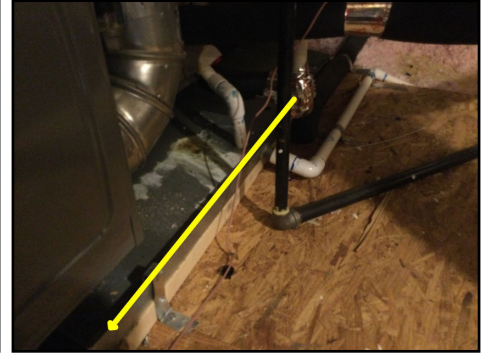
Water level detection device not present across drip pan
