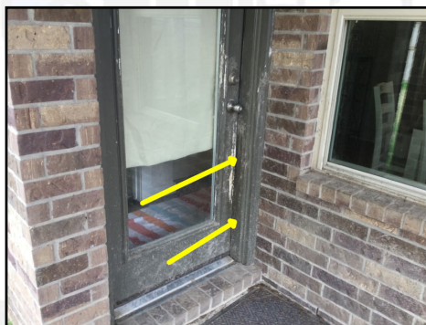
Damaged weather stripping observed along back door location
