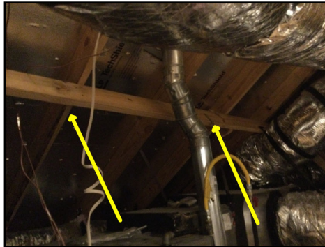
Purlin bracing not present across every 4' over attic furnace area (Recommend a building/framing contractor for further evaluation)
