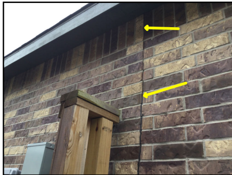
Areas along right expansion joint not sealed
