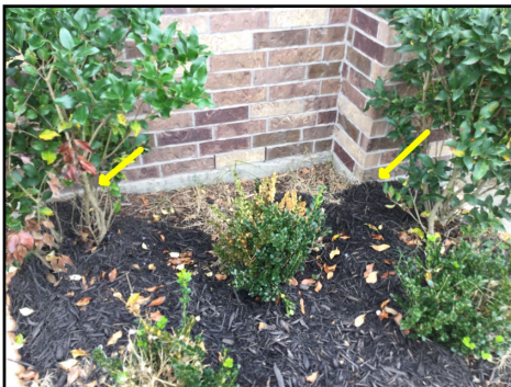
Soil to brick contact observed along front exterior wall (Recommend 4" or more slab exposure across all soil to brick areas per compliance)
