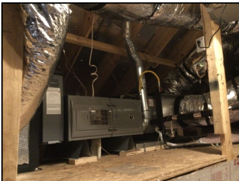
Attic furnace unit inspected
