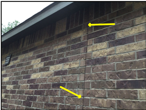
Expansion joint missing sealant along left exterior wall
