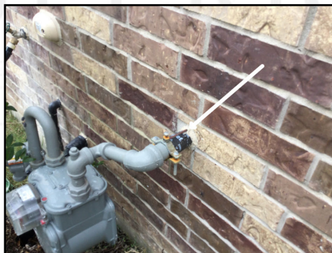
Bonding appears to be present around gas meter piping (This and bonding at grounding rod appeared to be only bonding visible during the inspection)
