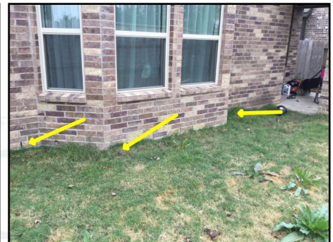
Soil to brick/siding contact observed along back exterior
