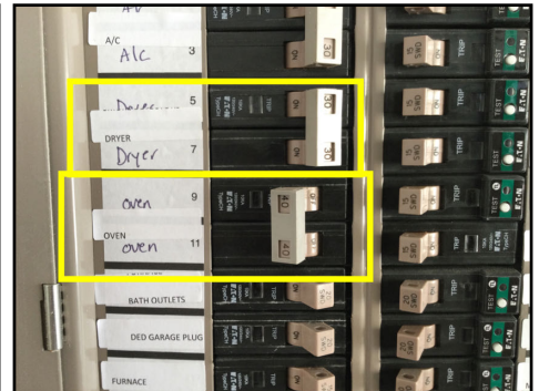
Oven and dryer breakers do not appear to be GFCI protected (Recommend an electrical contractor for further evaluation. FYI, Oven breaker was set to the off position prior to evaluation)
