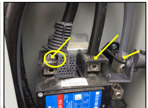
(Arrows) Anti-oxidant paste not present around service aluminum cables; (Oval) Cut/damaged wiring strands observed (Recommend an electrical contractor for further evaluation)
