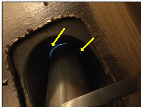
Daylight exposure observed around furnace flue piping penetration
