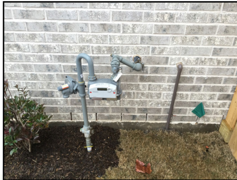
Gas meter located along right exterior
