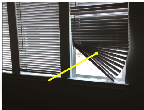
Upstairs game room window blind not functioning properly
