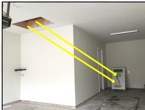
Exposed opening observed along garage attic (Ladder inside box was present along back wall during inspection)
