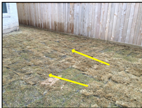
Water settling observed along back left swale
