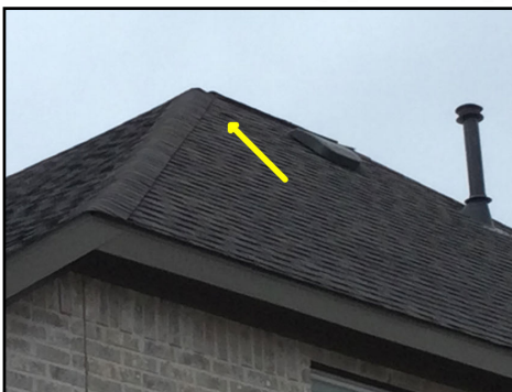
Lifted shingle along front right exterior
