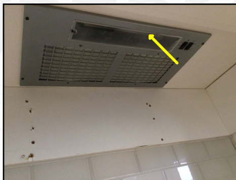
Kitchen exhaust vent lighting not functional
