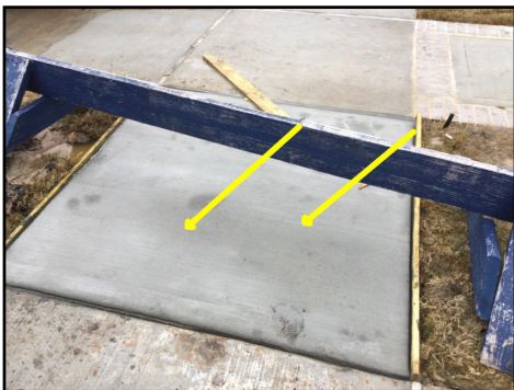
Previous repair noted at front walkway (Footprint noted along edge location)
