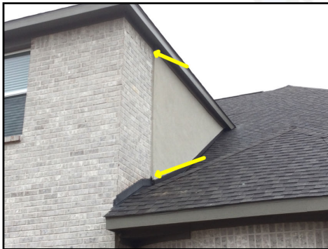
Exposed gaps observed along back middle left wall (Recommend a stucco contractor for further evaluation)
