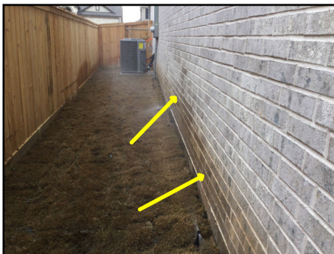
Various head(s) spraying along exterior walls (Recommend adjustments to spray away from exterior brick wall)
