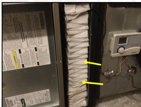
Filter dirty along media access location
