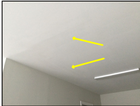
Previous repairs noted along interior garage ceiling
