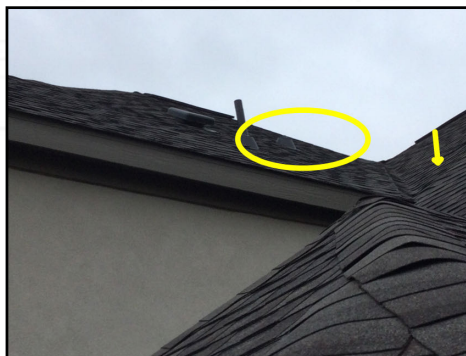
(Oval) venting appears to be below standard height over trim at back middle left; (Arrow) Protrusion observed near valley area (Recommend a framing and/or roofing contractor for further evaluation)
