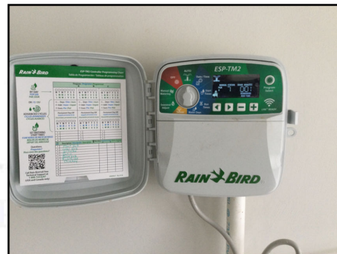
Interior garage irrigation console
