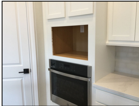
Microwave unit not present during inspection
