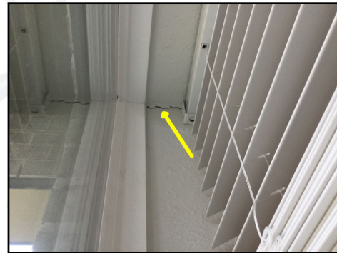
Drywall cracking observed throughout home (Downstairs living room top area pictured, as client should advise with builder regarding all cosmetic and drywall cracking areas prior to acceptance of property)
