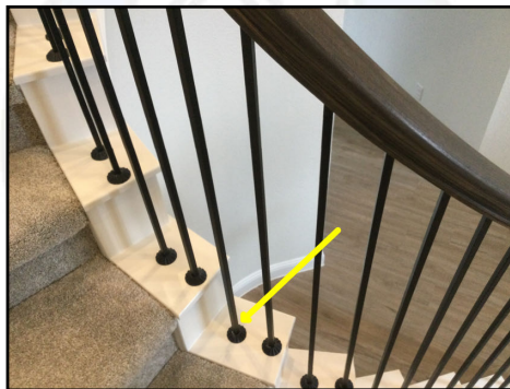
Loose baluster observed along handrail location (Recommend securing spindle along location)
