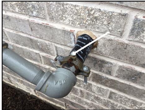
Bonding/grounding observed around gas meter piping
