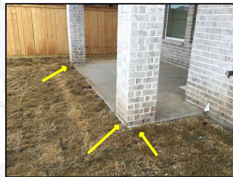
Soil to brick/siding contact observed along one or more exterior location(s).
