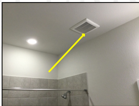
Unit not functional at upstairs hall bath
