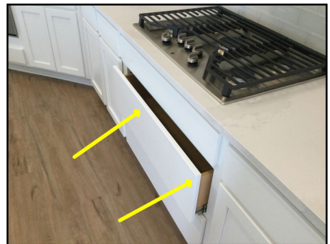
Kitchen cabinet not closing properly
