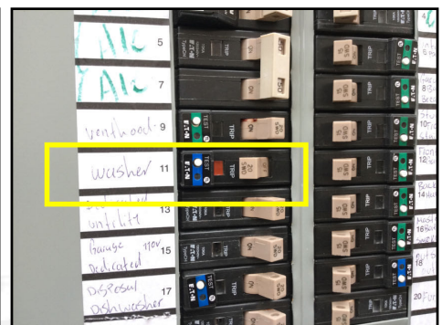
Breaker labeled for "Washer" does not appear to reset during evaluation
