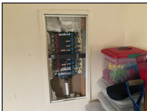
Right interior garage plumbing manifold inspected
