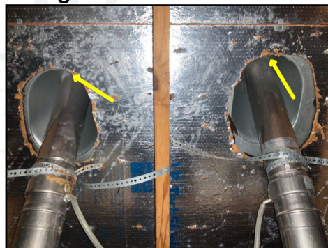
Daylight observed around both water heater flue piping penetrations
