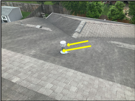
Sealant does not appear to be present around back flue piping (Piping does not appear to be proper height (3' above roof) per standards and recommend a plumbing contractor for further evaluation)
