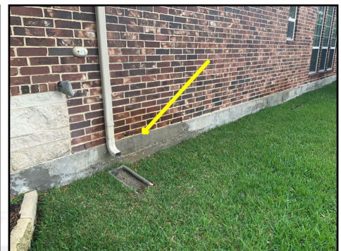
Various head(s) spraying along exterior wall(s).
