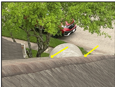
Debris damming observed along left and right connections (Recommend roofing contractor for further evaluation of coverings and all other respective components)
