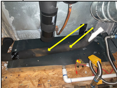
No P-Trap was visible on the condensate line and is required under current mechanical standards.
