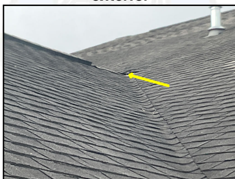
Exposed gap observed along back ridge
