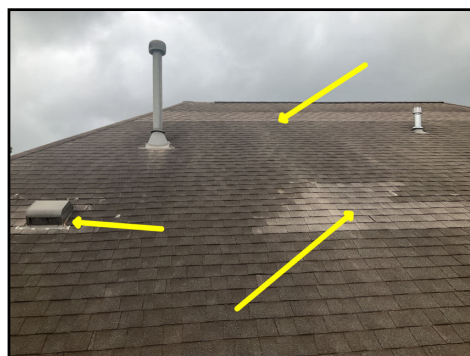
Potential previous repairs observed along back exterior
