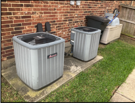
Left exterior condenser units inspected
