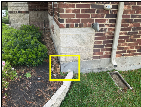
Foundation corner cracking observed along front right exterior
