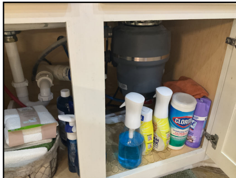
Kitchen sink disposer unit inspected
