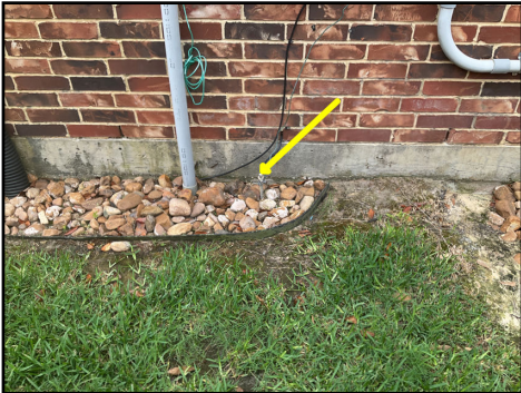
Ground rod does not appear to be fully installed into soil and/or improper ground clamp observed @ this time.
