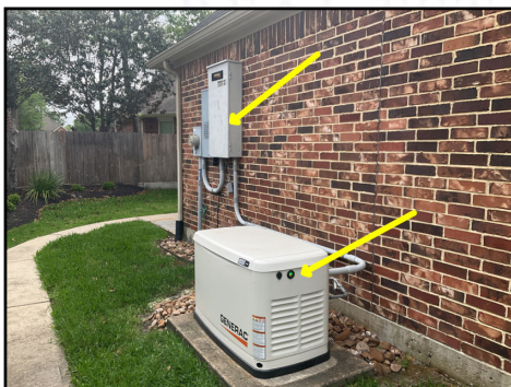
Left exterior generator and other respective components not part of the inspection
