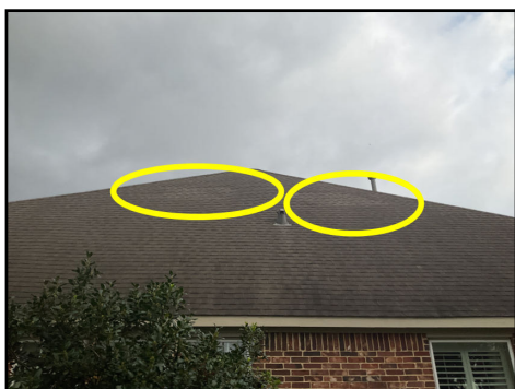
Potential previous repairs observed along right exterior
