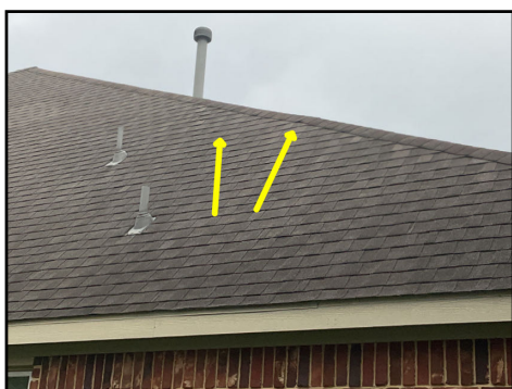
Lifted shingles across several exterior locations
