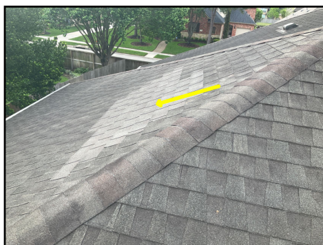
Potential previous repairs observed along back middle exterior
