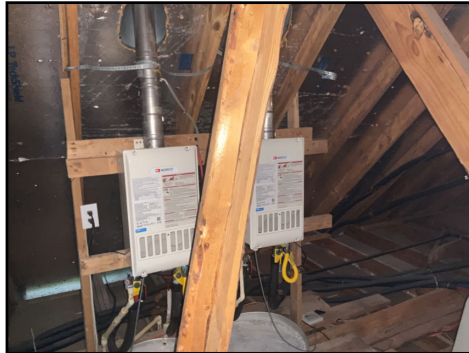
2 attic tankless water heaters inspected
