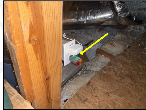
Attic receptacle does not appear to be GFCI protected
