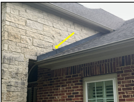
Exposed openings observed along front right exterior porch wall
