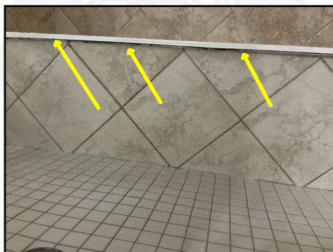
Damaged/organic growth observed along sealant under primary shower seat to wall
