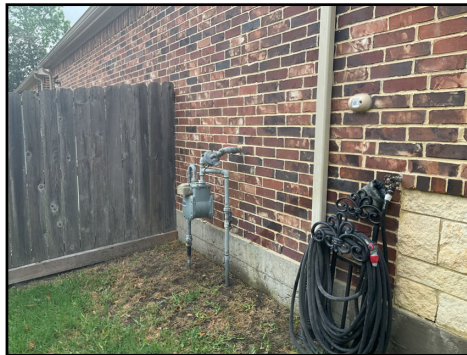
Gas meter located along left exterior
