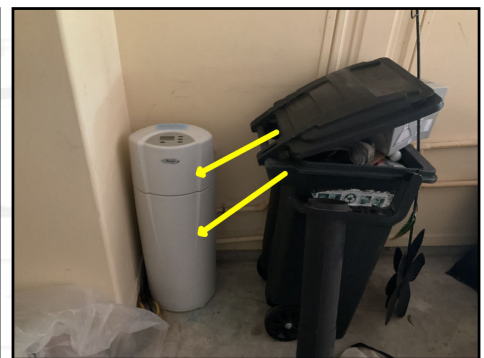
Interior garage water filter system not part of the inspection
