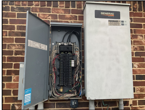
Disconnect/distribution panel inspected
