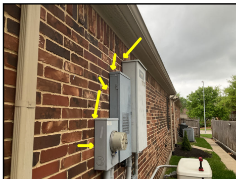
Sealant not present around left exterior electrical boxes
