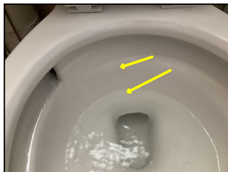
Hairline cracking appears t be present at right bathroom toilet
