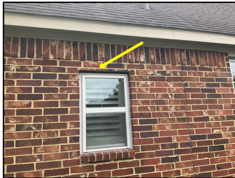
Weep hole(s) not present over right exterior metal lintil
