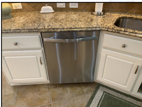
Kitchen dishwasher unit inspected
