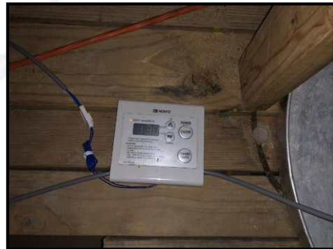
Both consoles read 130 degrees during the inspection
