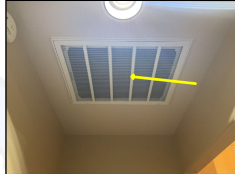
Filter(s) dirty inside home @ air return locations.
