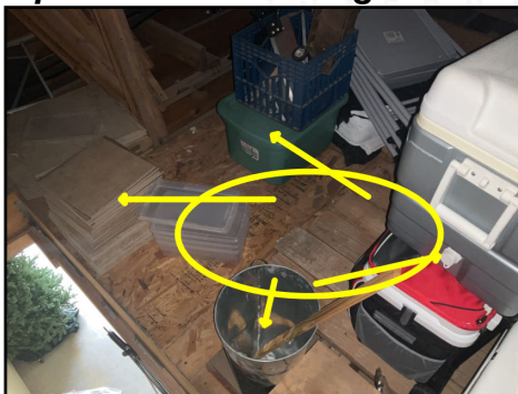
(Arrows) Storage observed across several interior attic areas; (Oval) Unsupported attic landing near opening (Safety hazards observed)
