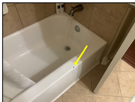
Gouged/chipped surface(s) observed across one or more interior tub surfaces.
