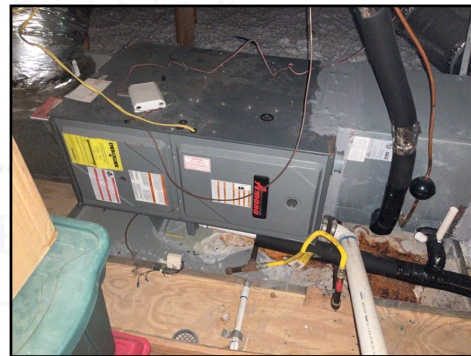
Right attic furnace unit inspected
