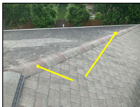
Significant granule loss observed across several shingle locations @ this time.
