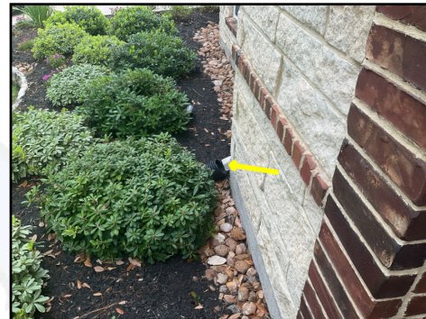
Disconnect observed between front gutter downspout and extension
