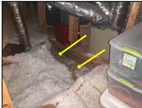
Deficient insulation depth observed at right of attic walkway platform
