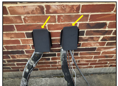
Exposed openings observed around left exterior a/c venting trim
