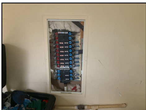
Left interior garage plumbing manifold inspected
