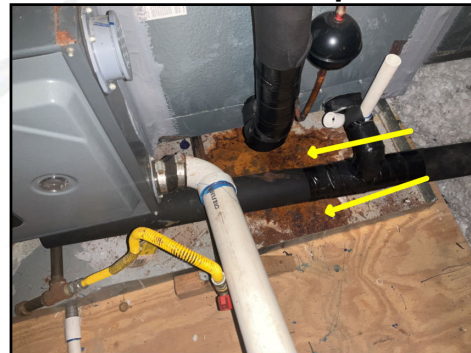
Significant rusting observed inside right attic pan
