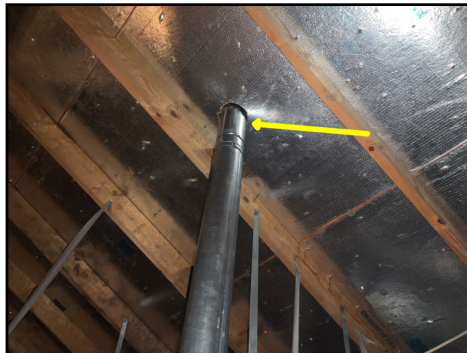
Back exterior furnace flue piping penetration in contact with roofing material
