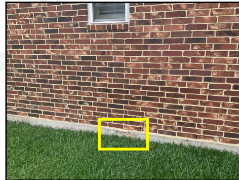
Potential previous foundation repairs observed along one or more exterior location(s).
