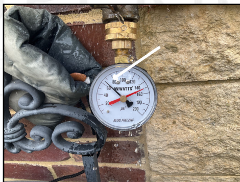
PSI measured between 66 - 70 range
