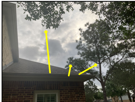
Trees/limbs appear to be close to structure.
