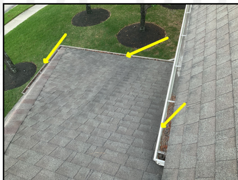
Dirt/debris observed across exterior covering and/or interior gutter system.
