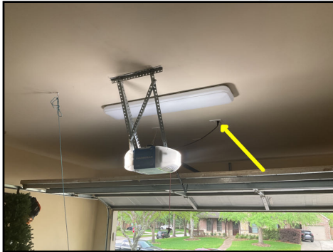
The GFCI (ground fault circuit interrupter) breaker not functional @ one or more location(s).
