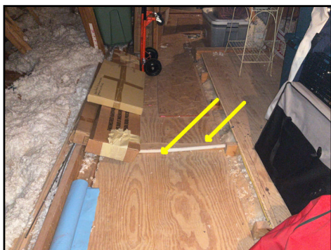
Drainage line appears over attic platform walkway (Safety/tripping hazard observed)
