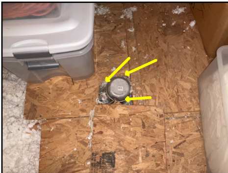
The attic insulation was observed to be covering the recessed lighting fixtures & should be removed from these areas to prevent overheating
