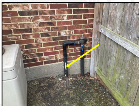
Damaged insulation observed around irrigation piping
